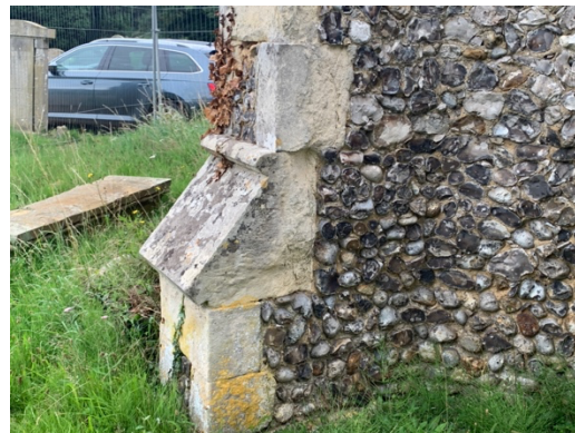
High soil levels covering plinth, B6.
