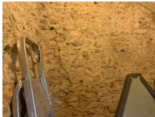
Cracks in west wall
