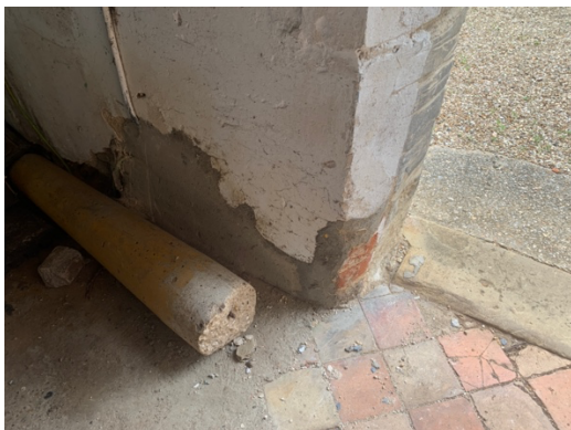
Damaged plaster and cement repair, D1
