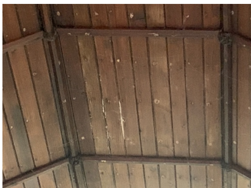
Ceiling, showing stains around nails and between boards
