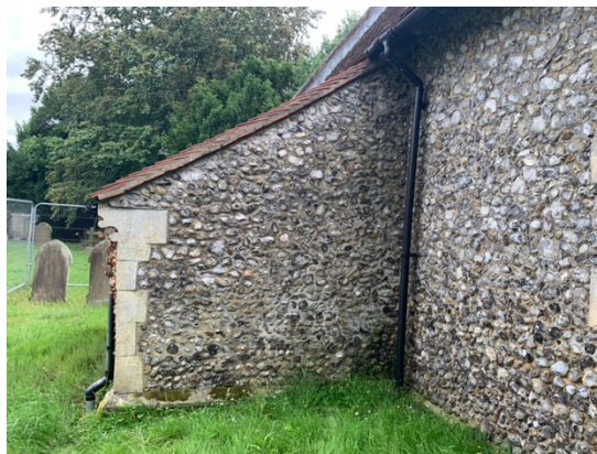
Damp in corner of Vestry
