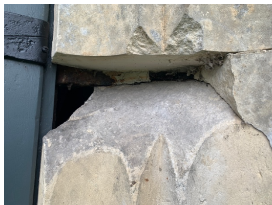
Rust jacking, D2, leaving a hole to the interior and an exposed pintle hinge.
