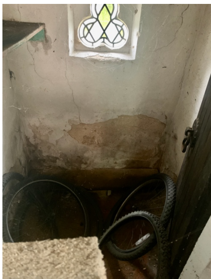
Damp damaged plaster, cupboard
