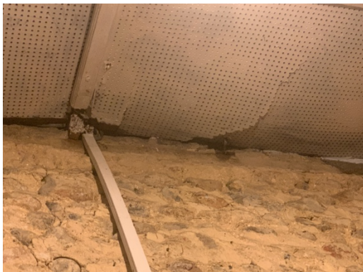
Damaged ceiling lining, Vestry
