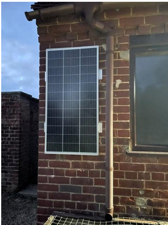
Exterior Solar Panel
