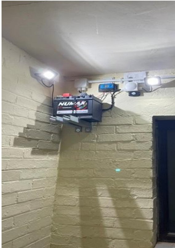
Toilet Light and battery store
