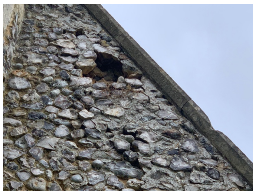
Loose and missing facings, east wall
