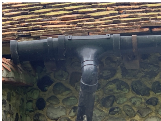
Poorly aligned PVCu gutters, north side
