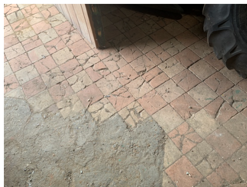
Damaged floor tiles and cement screed patch
