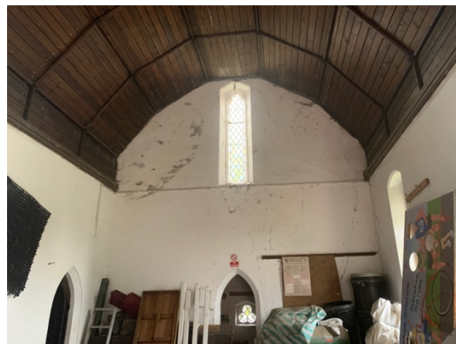
Damp at high level, north west side
