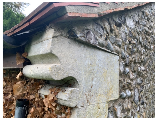
Misaligned flint facings, west side of Vestry
