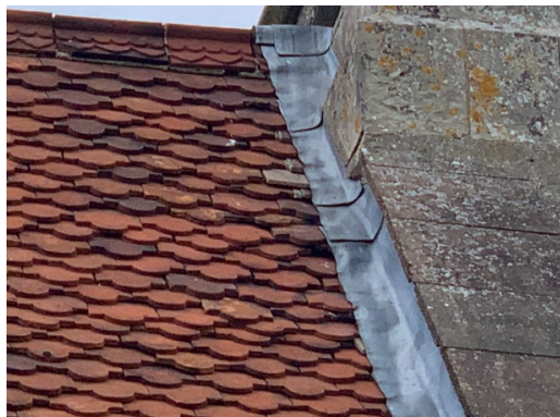
Chapel Roof, south east, poor lead flashing and slipping tiles at abutment
