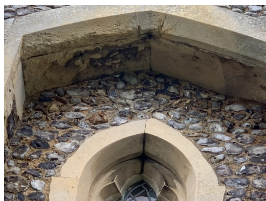
Water penetration through soffit of bellcote and top of E1.
