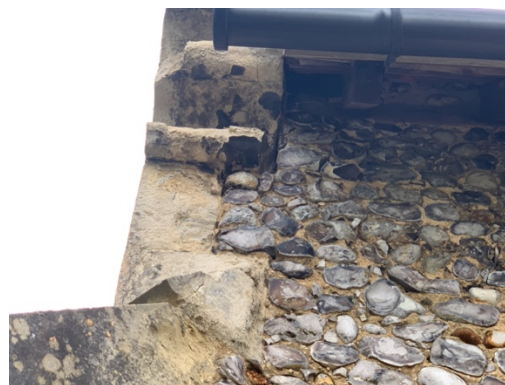
Eroded kneeler and quoins, south west corner
