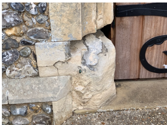
Damaged reveal to D1 due to rust jacking
