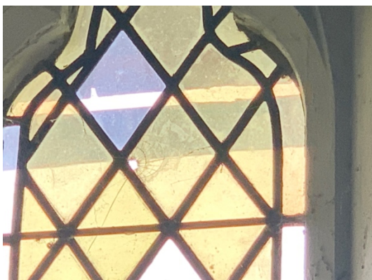
Hole in glazing of window S1
