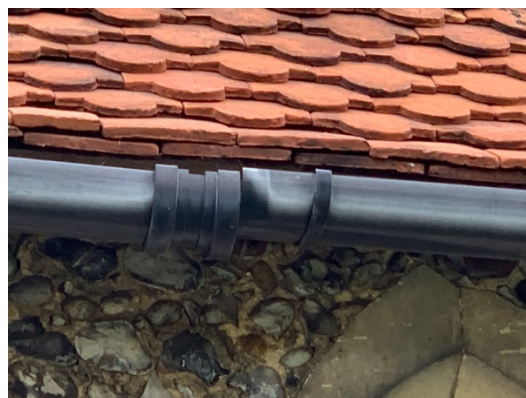
Joint failed, south side
