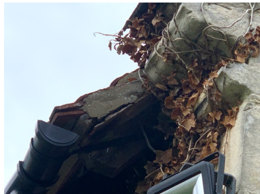
South east corner, showing poorly detailed verge
