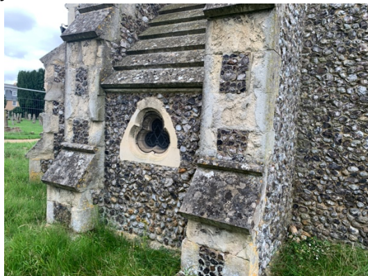
Erosion, B4 and B5. Cupboard roof
