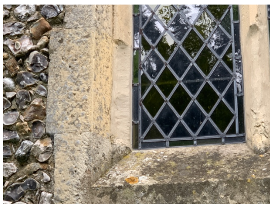
Poor plastic repairs, W1
